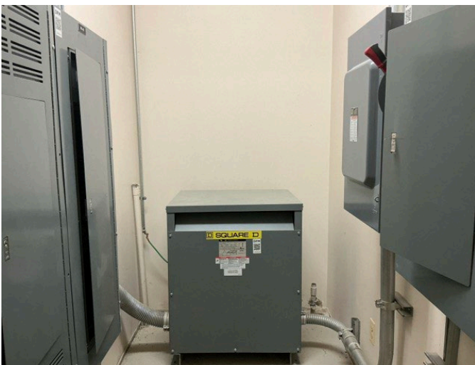
23 - SECONDARY ELECTRICAL ROOM
