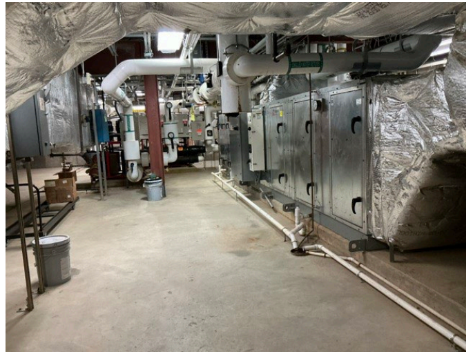
22 - MAIN MECHANICAL ROOM
