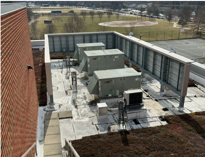
21 - ROOFTOP MECHANICAL EQUIPMENT
