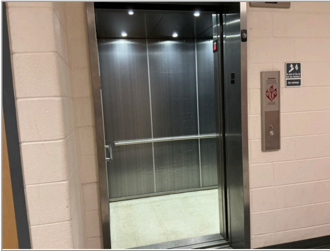
LOBBY LOOKING AT CABS (WITH DOORS OPEN)
